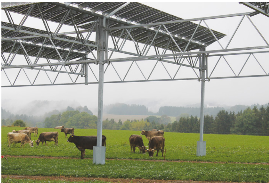
Source: BayWa r.e. AG, AgriPV above crops a) single row installation b) multi-row installation
