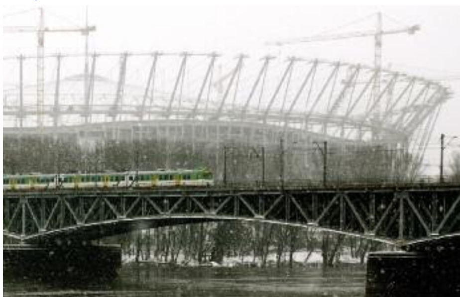
National Stadium in Warsaw, being built for UEFA EURO 2012 and a railway passage Photo by Michał Matera
